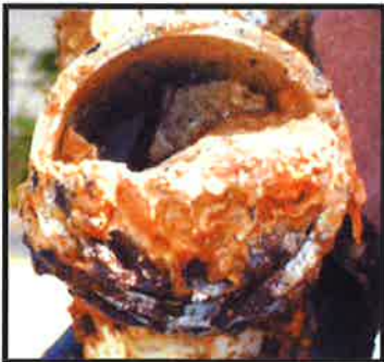
Grease found in piping
